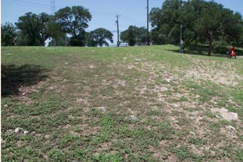
Mowed caliche sparse grass cover does not control erosion or reduce downslope flooding
